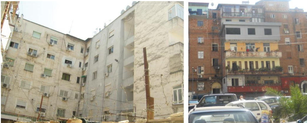
Figure 1. Building constructed after '90. Facade degradation.
